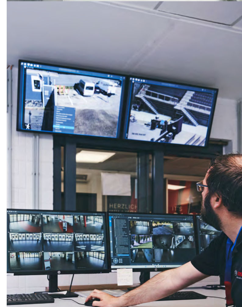
The individual cameras can be controlled in the control center
