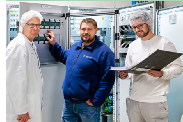
Project Manager Martin Hartmann (center) hands over the control cabinet to Technical Operations Manager Andreas Sepp (left) and Production Manager Martin Reischmann (right) from Allgäu Milch Käse eG
